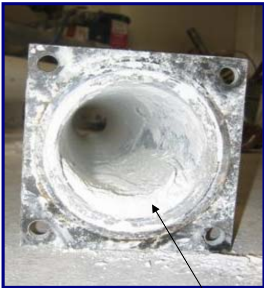
Loose sorbent settled out in conveying line
